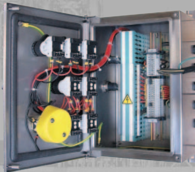
Stainless steel enclosure equipped and wired at the bottom of the box and on the door
