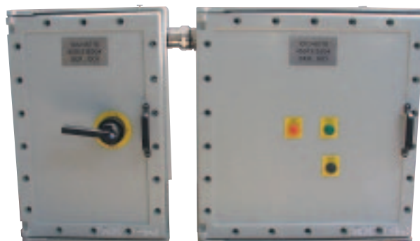
160 kW star-delta motor starter protected by MCB
