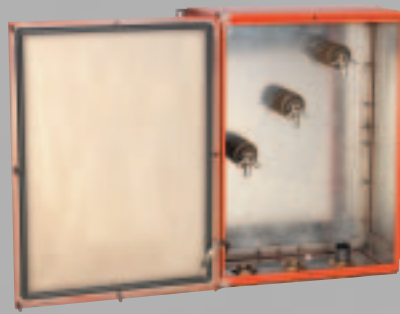
Medium voltage 10 kV
