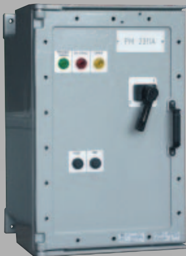
75 kW motor starter
