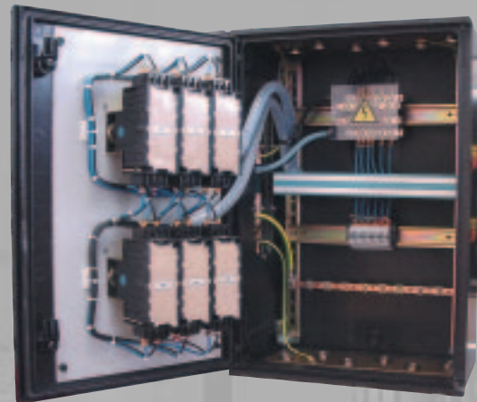
“Marina” distribution panel equipped with six two pole MCBs, mounted on the door
